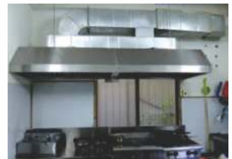
Kitchen Ventilation & Exhaust
